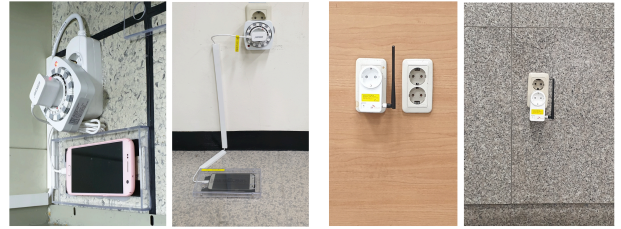
Figure 2: Snapshots of four actual sensors installed.
